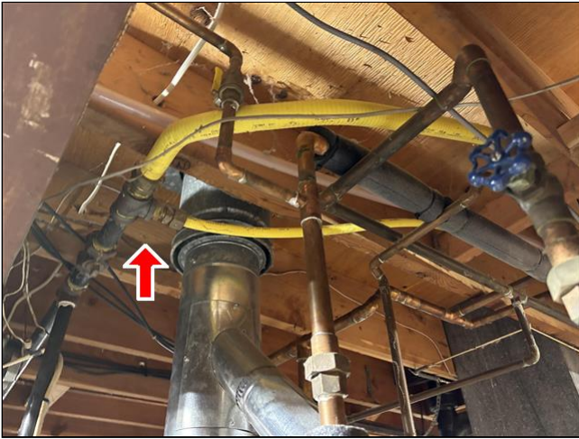
6.4 Ungrounded CSST gas line observed in home. The manufacturer of this product has updated the installation instructions to include/require grounding to the homes electrical system. When originally installed there was no requirements for bonding CSST gas lines. I attached the updated bulletin with the inspection report. Recommend a licensed electrician perform work. It should be noted that this fix is for lightening protection of gas lines. In most cases the update can be completed quickly.
